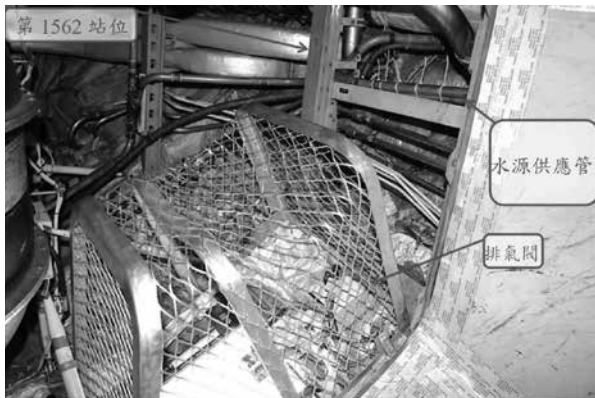
The water supply pipe passing close to the OFV. [Reproduced from the Official Report]
